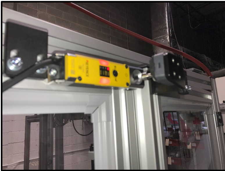
PHOTO 12 - Door locking limit switch
